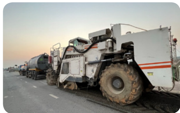
Cold In Place Recycling projects supplied by ADCo - Vinh Phuc (2023) Highway 13, Vietnam
