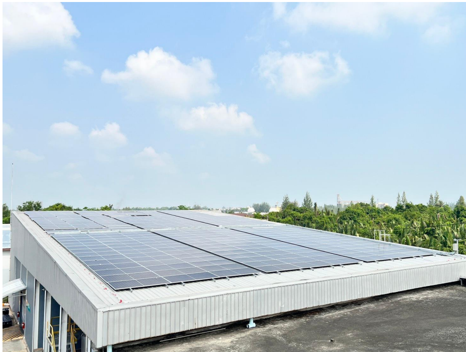
Solar Roof at Surat Thani Plant
